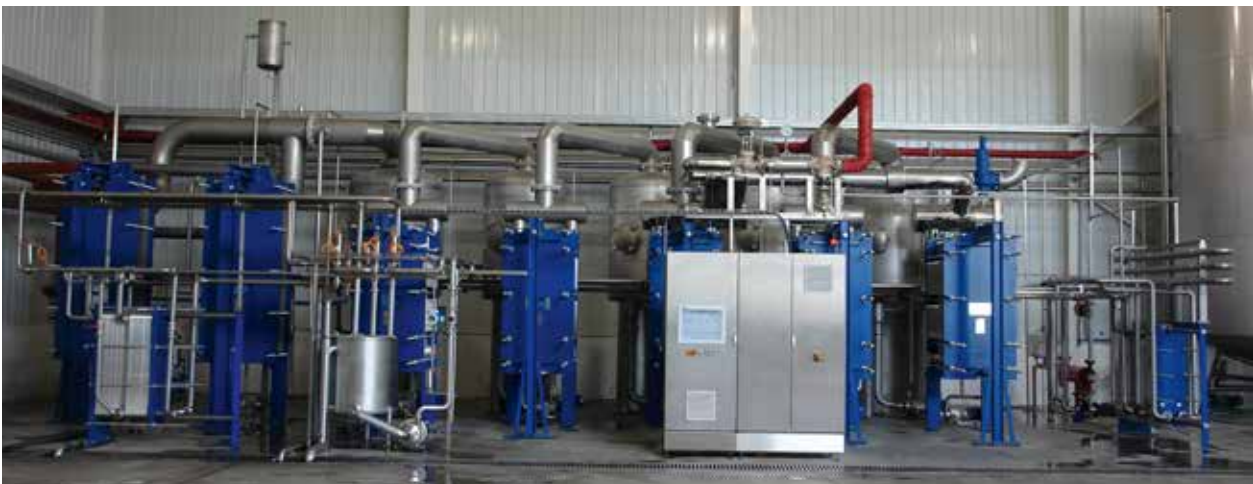
5-stage SIGMASTAR® 90V Evaporating Plant with thermal vapor compressor for apple juice - evaporating capacity 20,000 kg/h
